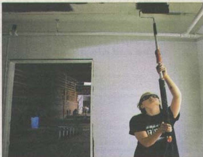
Ashley Guy, 13, of Virginia Beach and a member of the Virginia Youth Symphony Orchestra, volunteers to help paint the backstage area. Ashley said she and her parents, Robin and Phil Guy, spend nearly every weekend working on the building.
